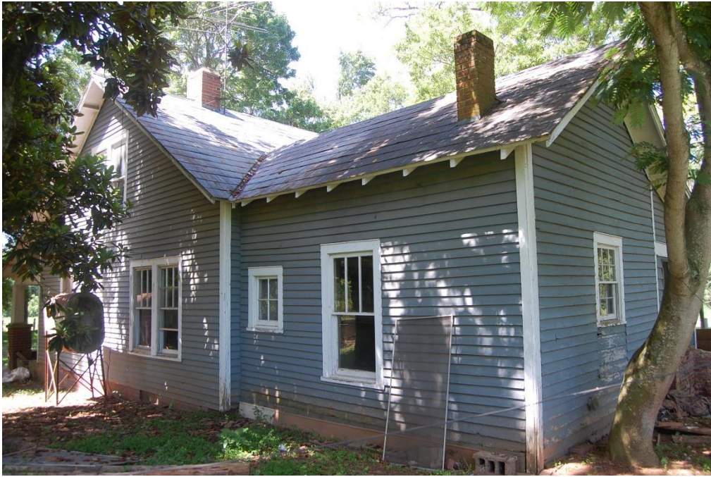
Latta Family House, Side (West) Elevation of House and Kitchen Wing and Rear (North) Elevation of Kitchen, Looking Southwest.
